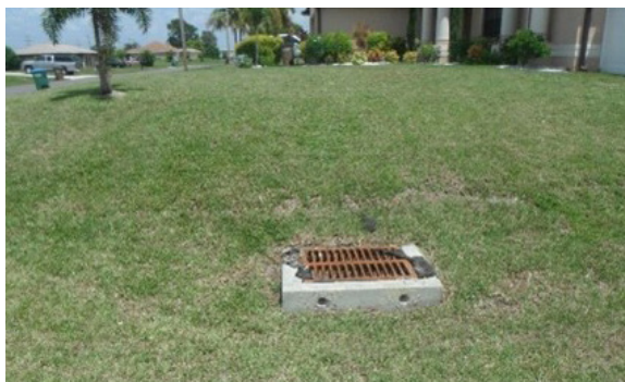
Raised Grate Inlet
